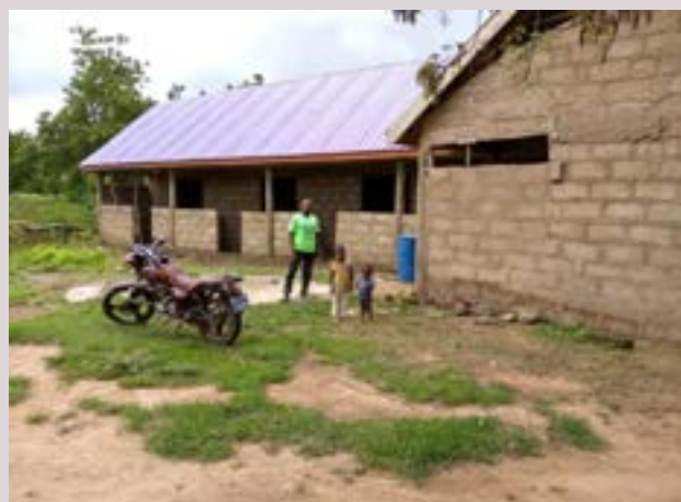
A 3 Bedroom house being put up by Mr. Hudu Dramani of the Sibelle community seed production group in the Sissala West district.
