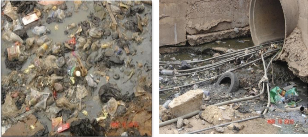
Plate 2: Sanitary condition (left) and illegal connections through wastewater channels (right) at Chorkor
