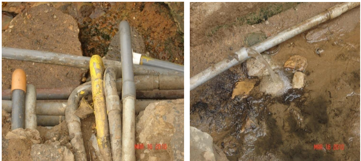
Plate 3: Illegal connections, leaked and burst pipelines at Chorkor
